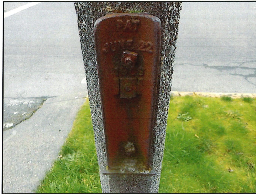
Figure 26. Close up of the broken bracket that was observed on three out of the five Mail Posts.
