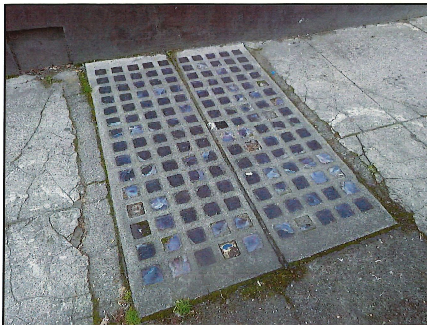
Figure 82. Feature 1, sidewalk vault light along the west side of S College Street.
