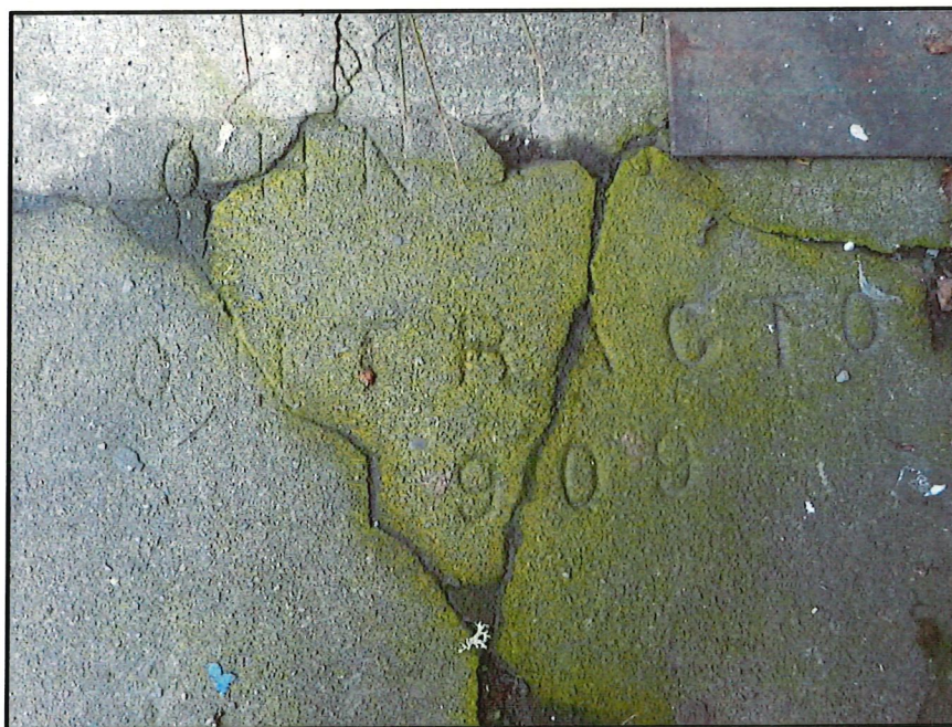
Figure 37. PS 25, located on the northern side of E First Street.
