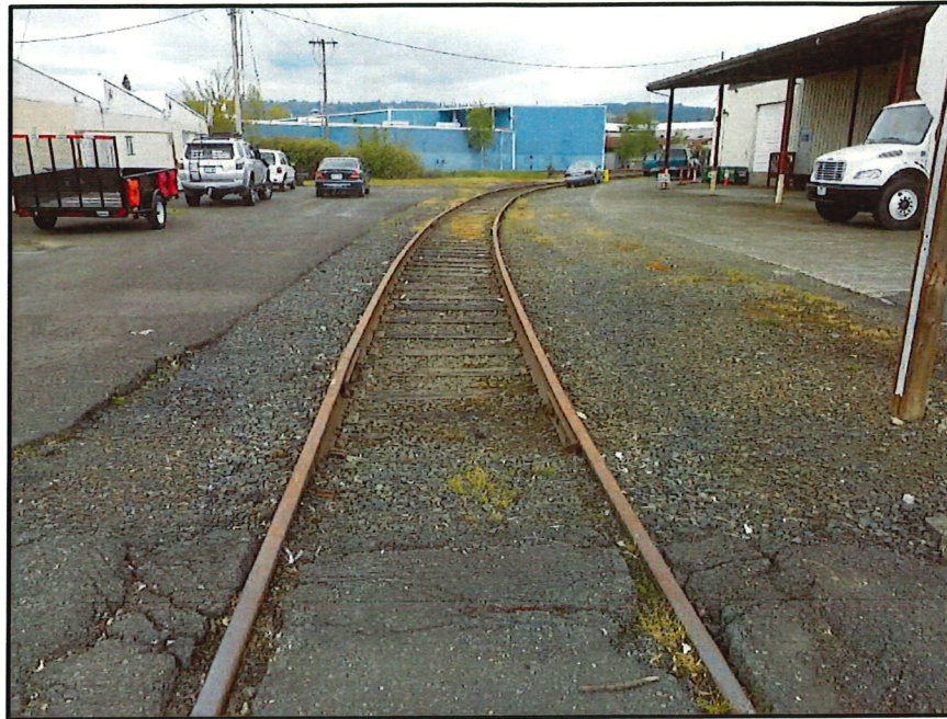
Figure 77. Northern terminus of the railroad track, looking north from the intersection of E Franklin and N Blaine Streets toward their intersection with the still operational tracks (in background).
