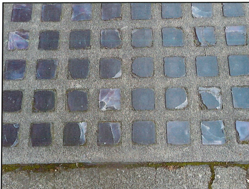
Figure 83. Close up of the amethyst glass prisms that comprise Feature 1, the sidewalk vault light along the west side of S College Street.
